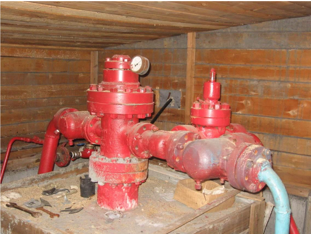
Figure 3.9. Wellhead of the Byelii Yar 1-R borehole (Photo by David Banks)
