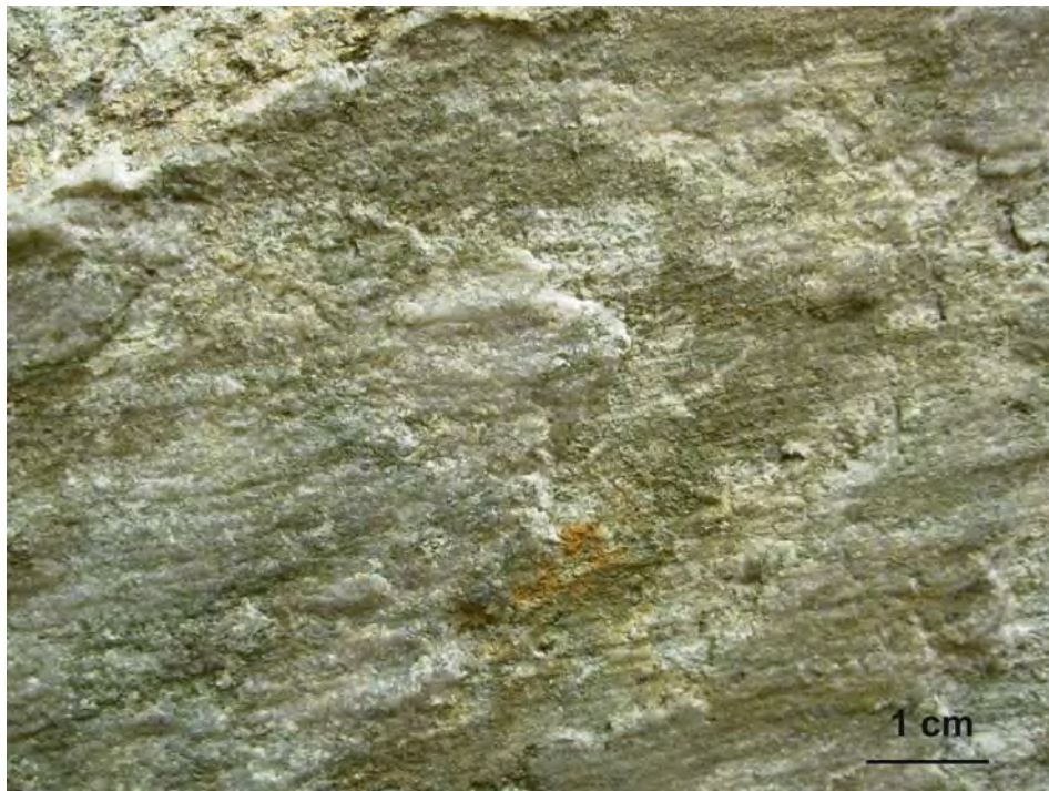
Figure 42. Illustration of the striated surface of a sinistral fault (strike/dip 285/46; pitch: 20W) which extends several meters at locality “Sportsplassen, Jomfrubråtveien”.
