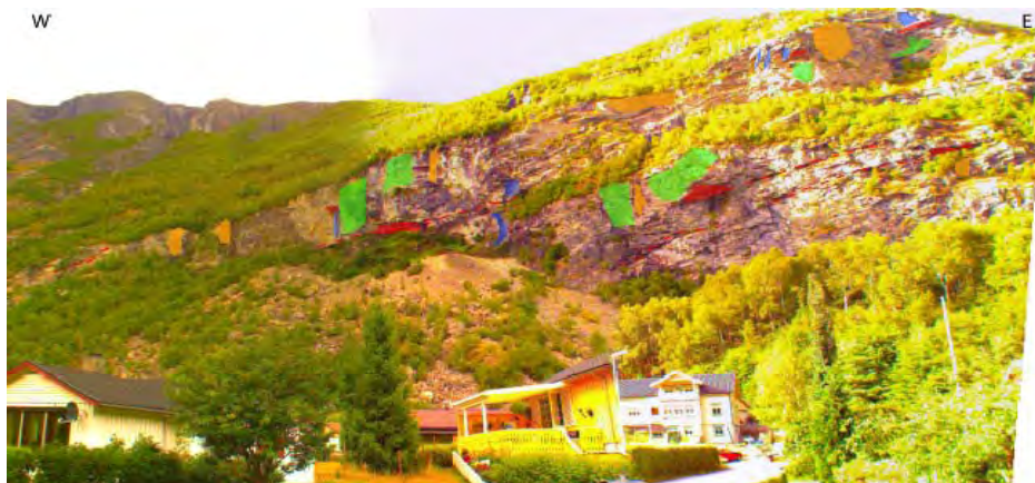
Figure 15: Panoramic view of the cliff with some examples of the main discontinuity sets (red=J1, blue=J2, green=J3, orange=J4).
