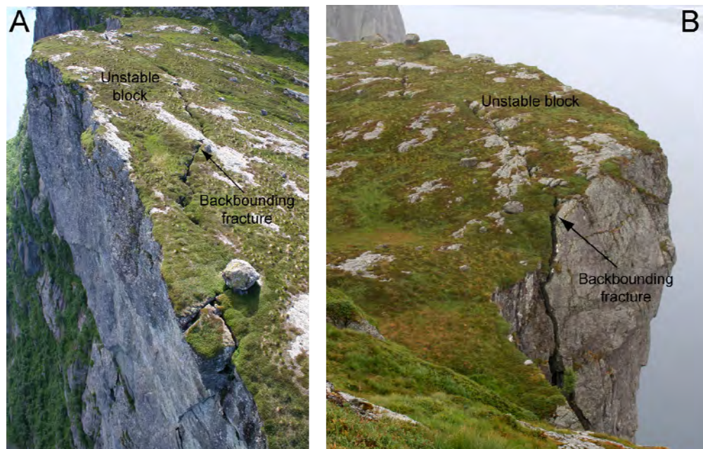
Figure 24. Airphoto-view of Lifjellet west showing the overhanging character of the cliff in front of the crack (after Böhme et al., 2011)
