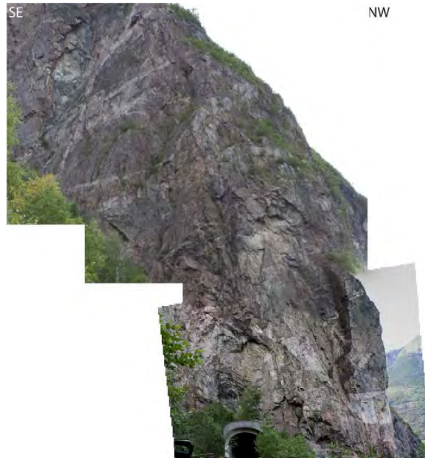
Figure 17: Panorama of the cliff overhanging the old national road tunnel. Only the upper part of the cliff has been scanned.
