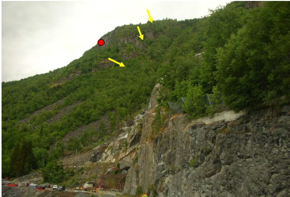
Figure 59. View of Anhovden from the south. Arrows indicate the weak open structure discussed above. The western entrance of the new tunnel, which was built because of the high rockfall- activity, is also shown. The red dot could represent the centre of the source area for the small rockslide in Figure 53.
