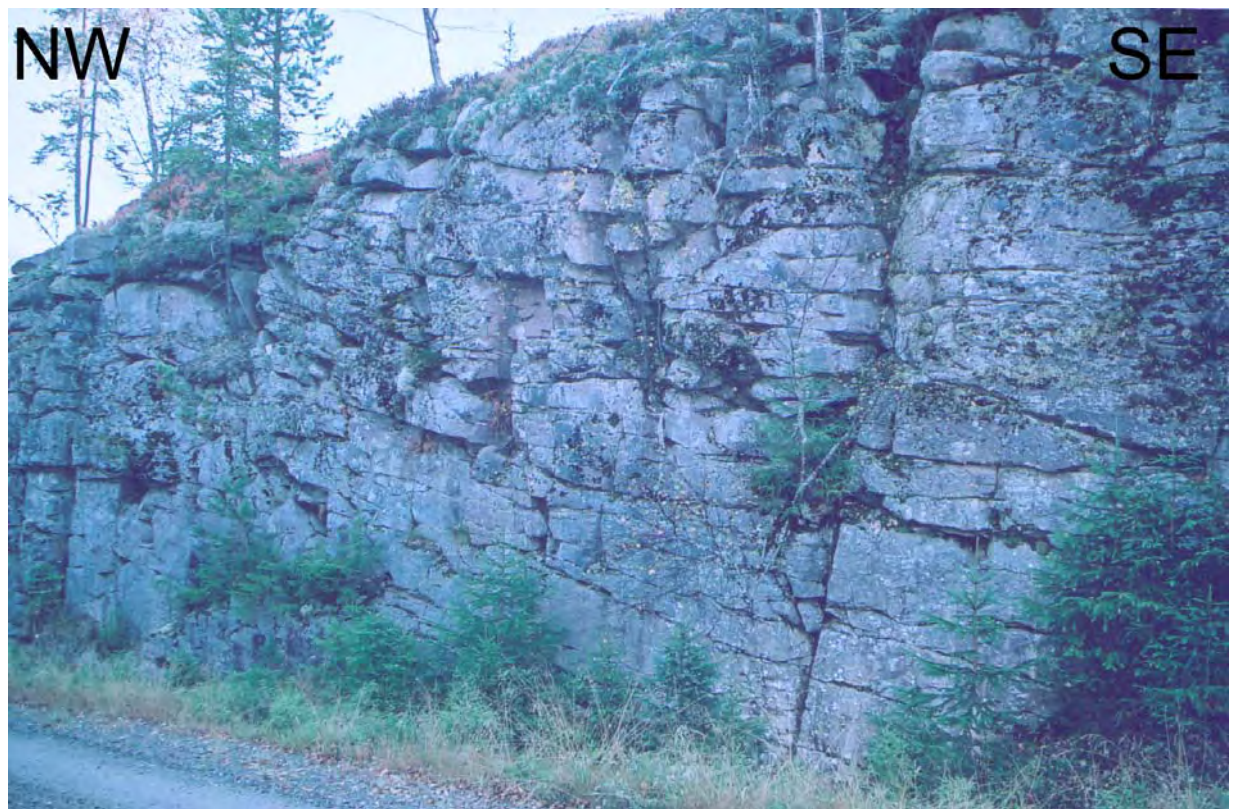
Figure 17. High density of joints at site 21, with both flat lying and steep joints. N-S (the wall on the picture) and NE-SW to ENE-WSW are the predominant trends of the large step joints.
