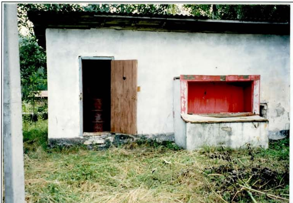
Photograph 6: One of the buildings in the chemical storage area. Several barrels inside the building were sealed and not sampled. Lit II-2 was taken from an open drum inside this building.
