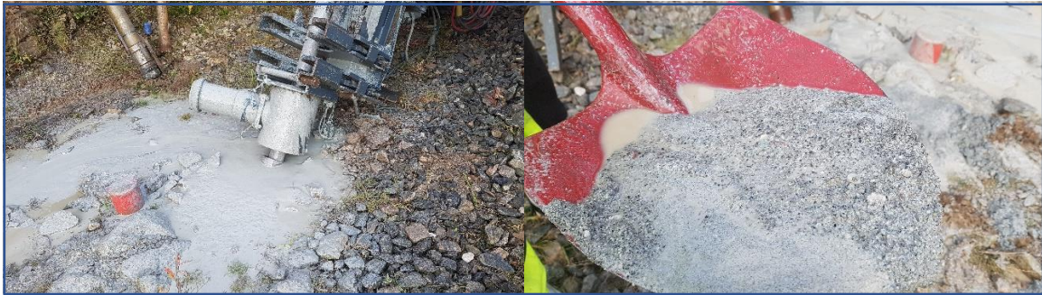
Figure 63. Reopening of Bh2. Clay (?) and sand were flushed out of the borehole.
