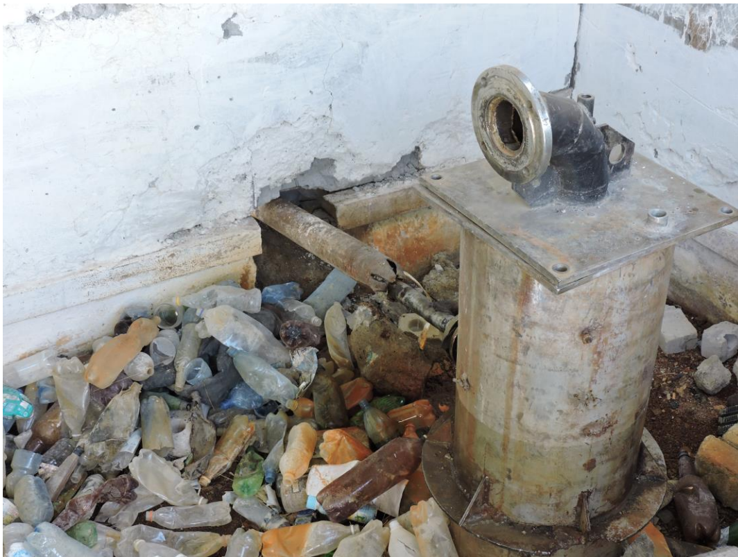
Figure 5.1 Bazanovskii borehole well head. The discharge pipe passes through the rear wall. (Photo by David Banks)
