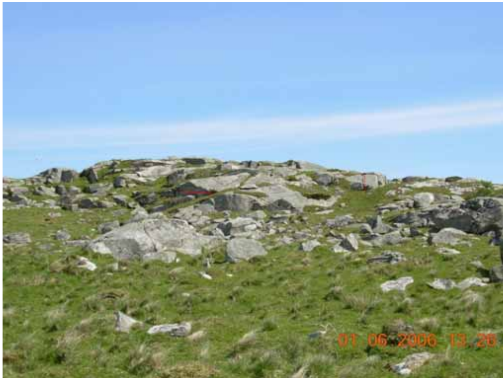
Figure 6.29. View to the NE of the outcrop at site 20 with the vertical joints striking NE-SW; here, they are linked to vertical joints striking NW-SE to form a perpendicular system of joints (the two sets are underlined in red).
