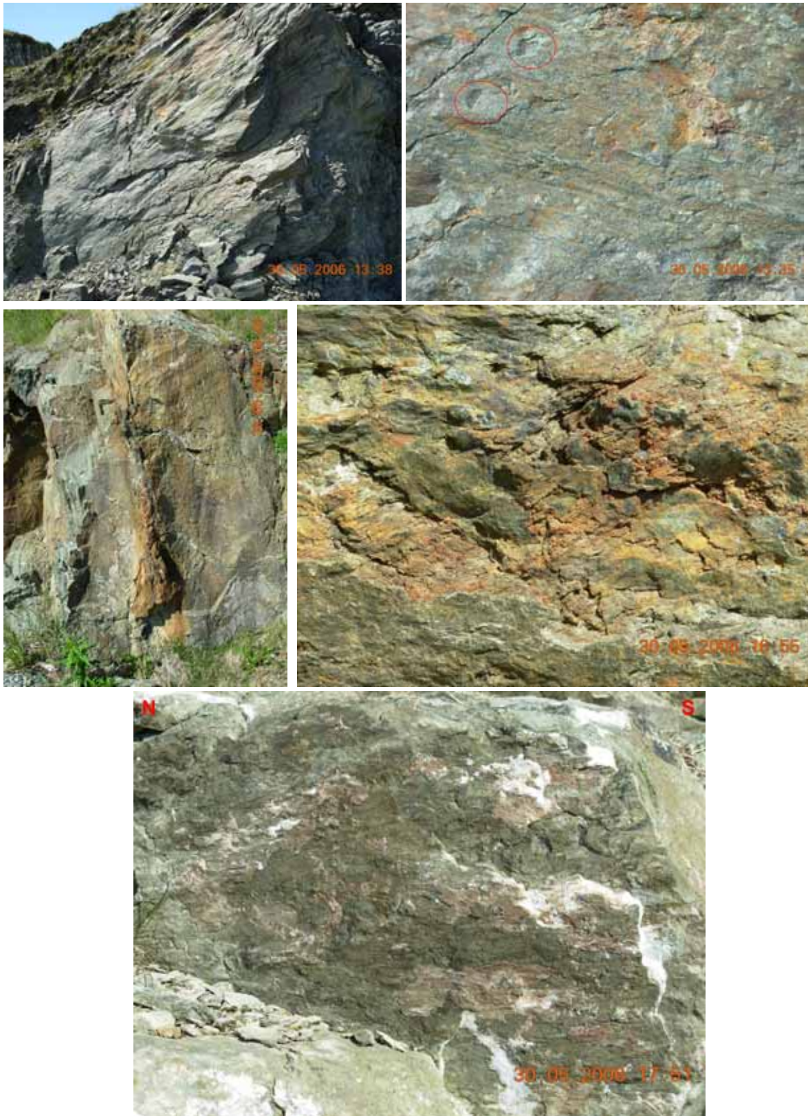
Figure 6.14. Examples of strike-slip faults. Top left: view to the W of a large NE-SW strike-slip fault plane and top right: of the left-lateral striae and the lunate fractures observed on the plane (site 8). Middle left: NNE-SSW strike-slip fault and its damaged mineralized zone and middle right: the strike-slip striae on the same plane (site 10). Bottom: horizontal calcite steps of a NE-SW left-lateral fault (site 11).
