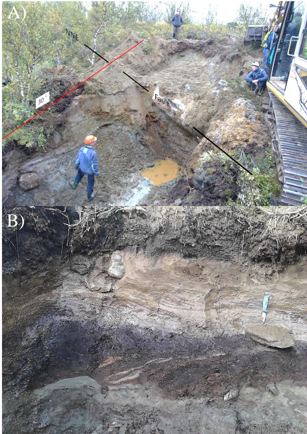
Fig 5. A: Trenching transverse to fault scarp associated with the Masi Fault System in the Stuuragurra Fault Complex, just north of Mási (7 in Fig. 3). Up thrown part of bedrock from the reverse fault is exposed in the central part of the photograph. The hanging-wall or fault plane is dipping c. 50° to the right (ESE). Fault breccia, visible in the central part of the photograph, is in contact with the bedrock hanging wall. The fault breccia is produced, pushed, and injected during the fault event into the sediment overburden, with deformation and burial of sediments and organics as a result. B: Partly deformed surficial peat overlying deformed layered lacustrine sand, buried peat and till and glaciofluvial sediments in the 2018-trenching at Mási (7 in Fig.3).
